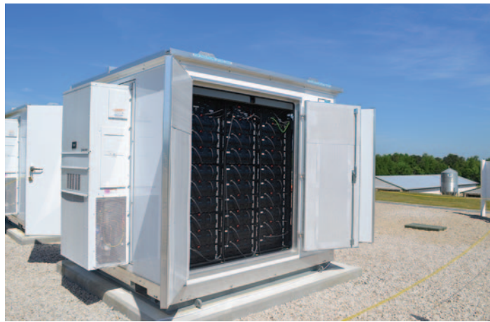
This 250kW/735kWh battery storage system is owned by North Carolina's Electric Cooperatives, in partnership with South River EMC.
