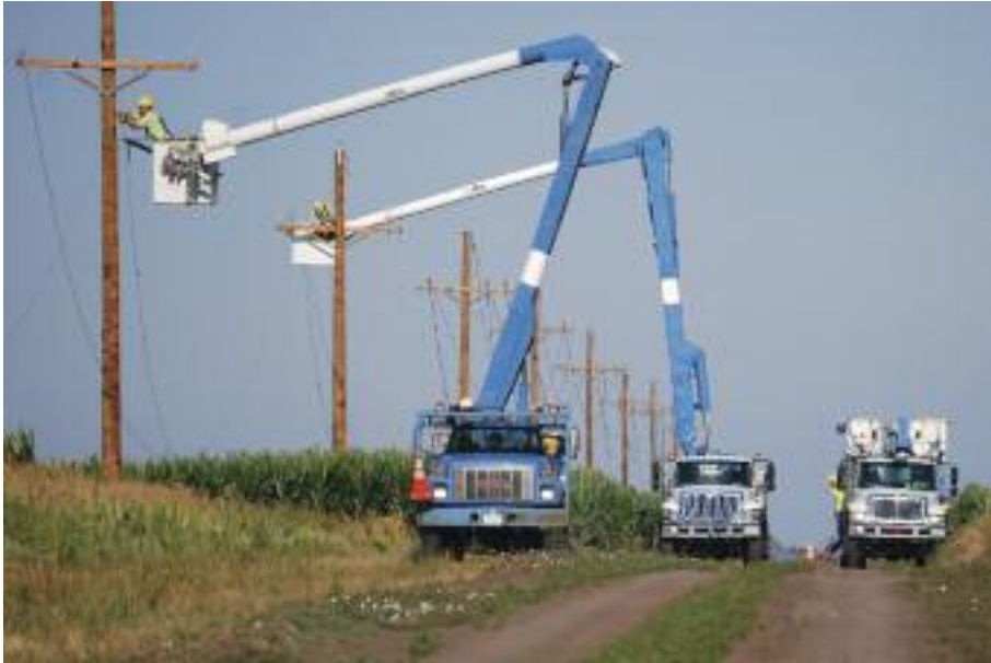
Above: Norris Public Power District crews work together to build a power line in Gage County.
