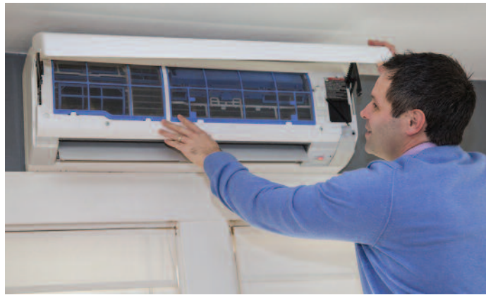
A homeowner shows off his energy efficient ductless heat pump. Photograph by Marcela Gara, Resource Media
