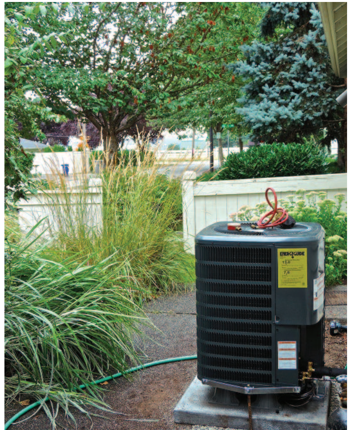
An air-source heat pump compressor located outside the home can distribute hot and cold air through your existing duct system. Photograph by Peter Stevens
