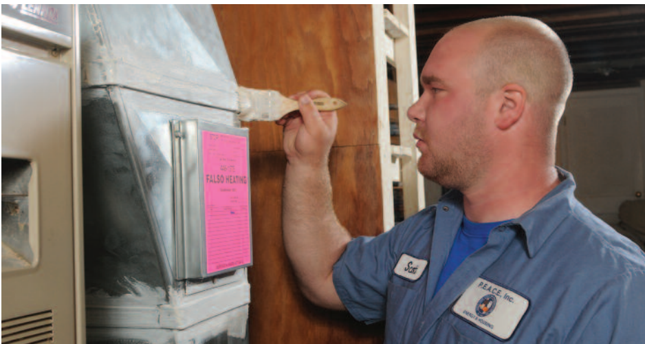
Mastic can be used to seal small gaps and leaks in your ductwork. Photograph provided by Weatherization Assistance Program
