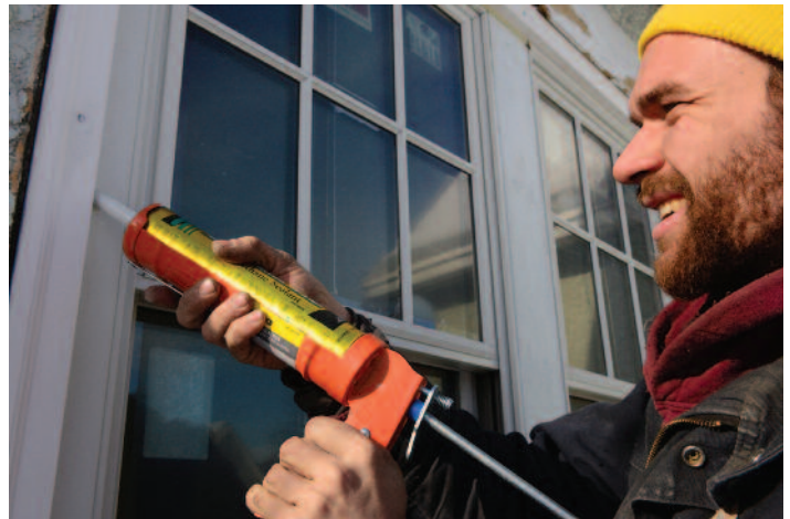
Caulking seals air leaks around existing windows as well as new windows. Photograph provided by rareformproperties.com
