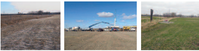
Left to right: Land prior to using composite matting, with matting in use, and after matting.
