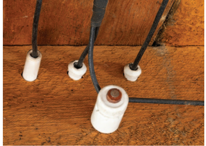
If household insulation is installed over knob and tube wiring, a fire is just waiting to break out.
