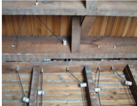
Knob-and-tube wiring in a 1930 home. Photograph by Laura Scudder
