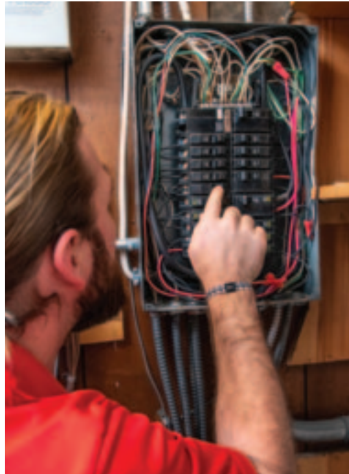
Ask your home inspector if the electrical panel can accommodate new appliances you might want to add. Photograph by Mark Gilliland, Pioneer Utility Resources
