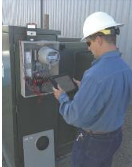
Many lineworkers use tablets to perform their duties.
